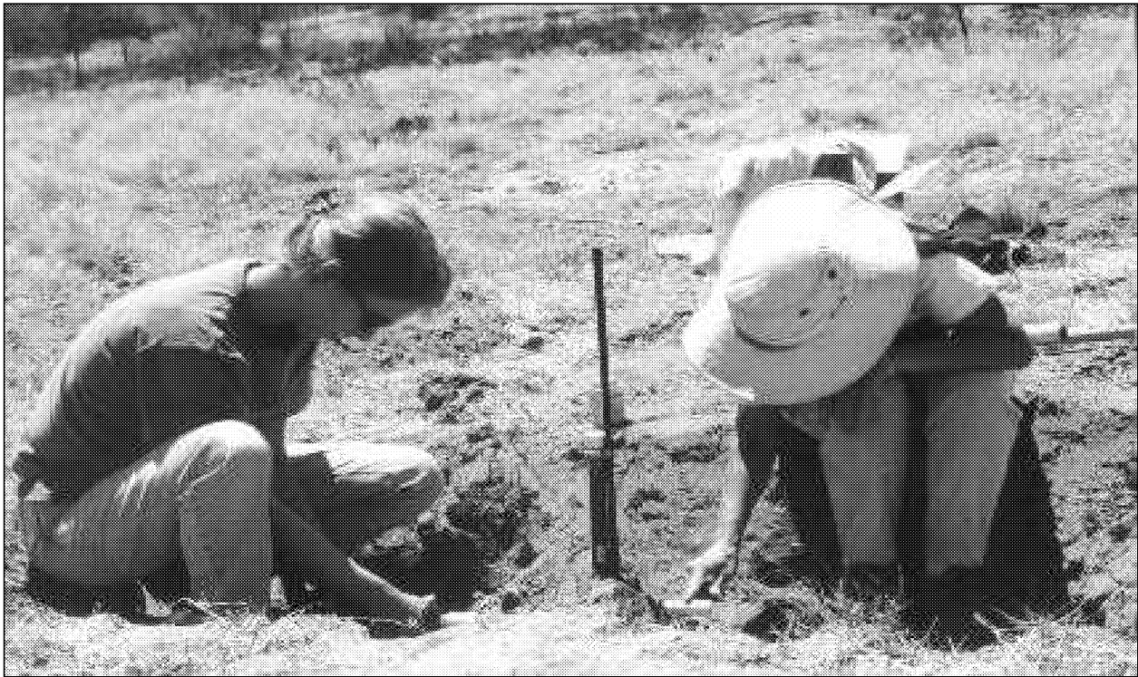
Figure 17. Rincon Institute Staff installing irrigation control valves at the Llewellyn Revegetation Site. 98-062WPF
