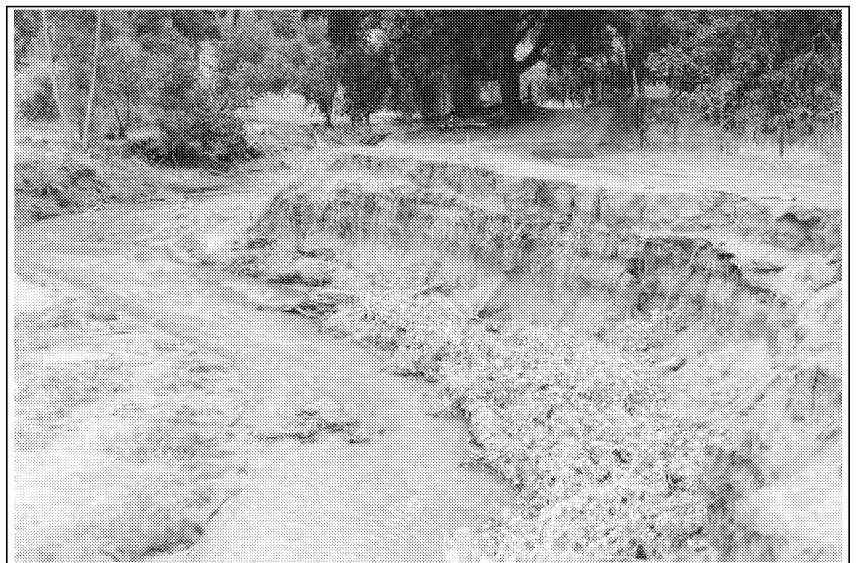
Figure 11. Site of potential road failure due to bank erosion, Canyon del Muerto. 96-0025WPF
