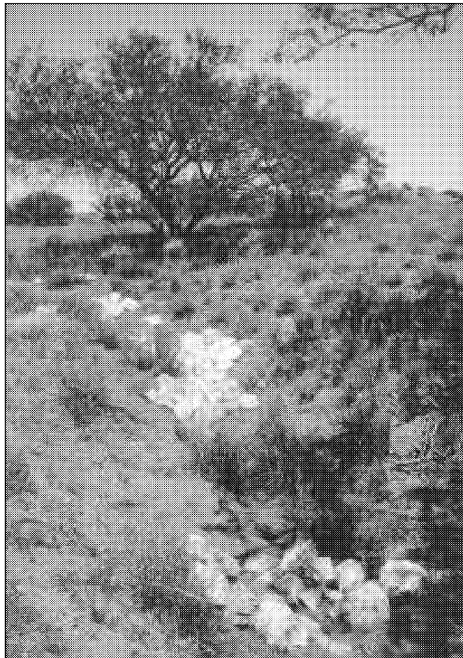
Figure 15. Headcut treatments in Oak Tree Canyon designed to decrease flow velocity and energy. 97-034WPF
