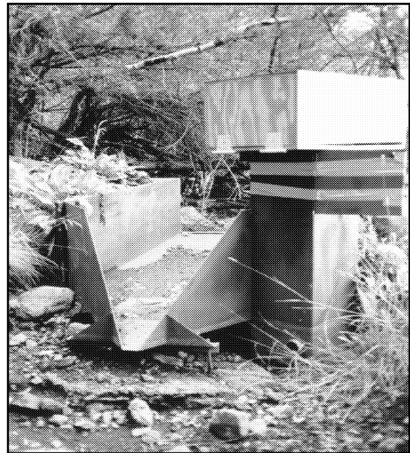
Figure 10. Flume installed to measure stream flow at Hart Prairie. 96-0019WPF.
