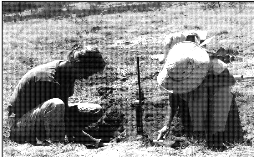
Figure 18. Rincon Institute Staff installing irrigation control valves at the Llewellyn revegetation site. 98-062WPF
