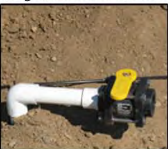
Flush out valve
