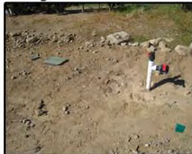
Flush out valve & valve boxes to access main line
