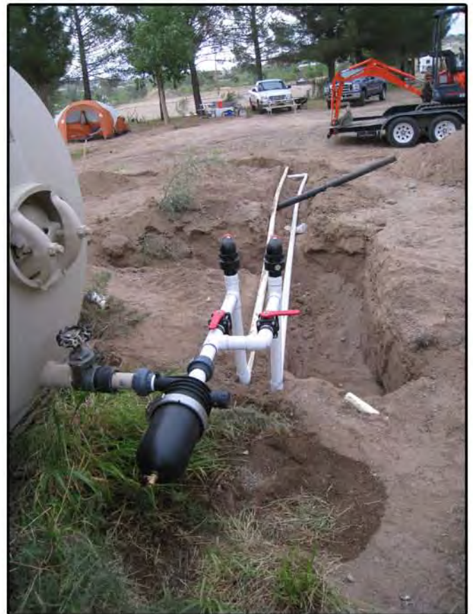
Irrigation Main control valves and filter setup
