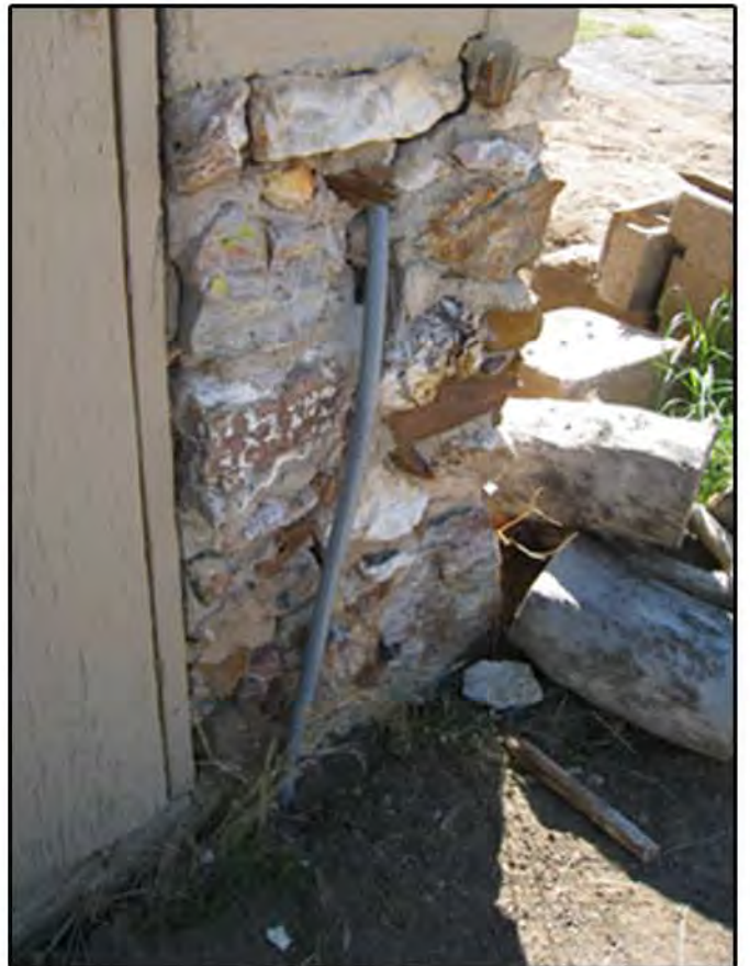
Electrical conduit for irrigation timer
