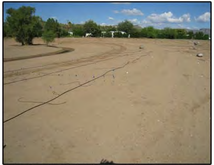
Irrigation PVC lateral lines with emitters around the wetland and pond to water cottonwood/willow habitat
