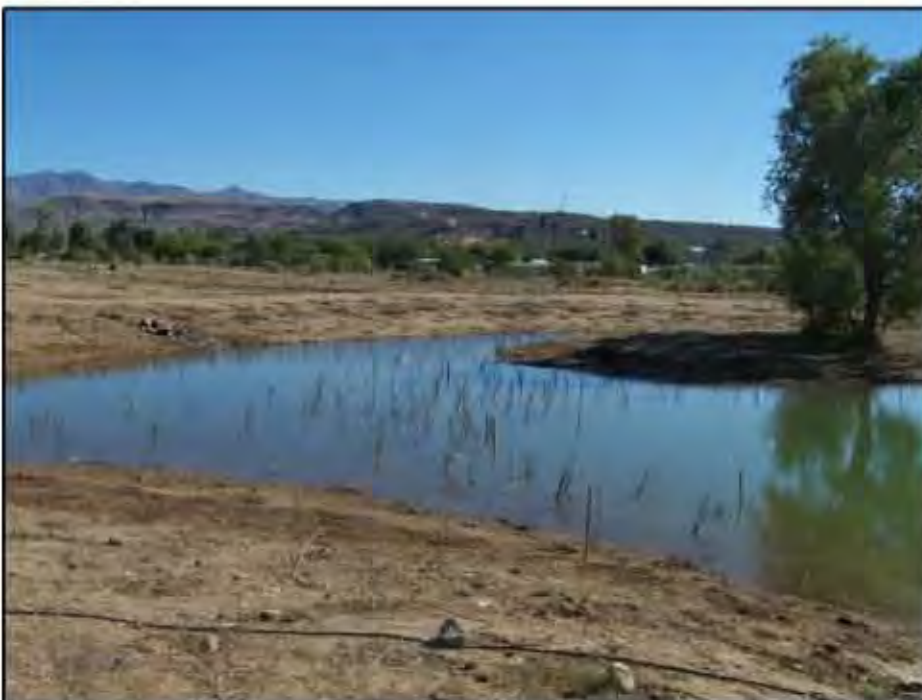
Completed planting of wetland and transitional zone on the north side of the pond
