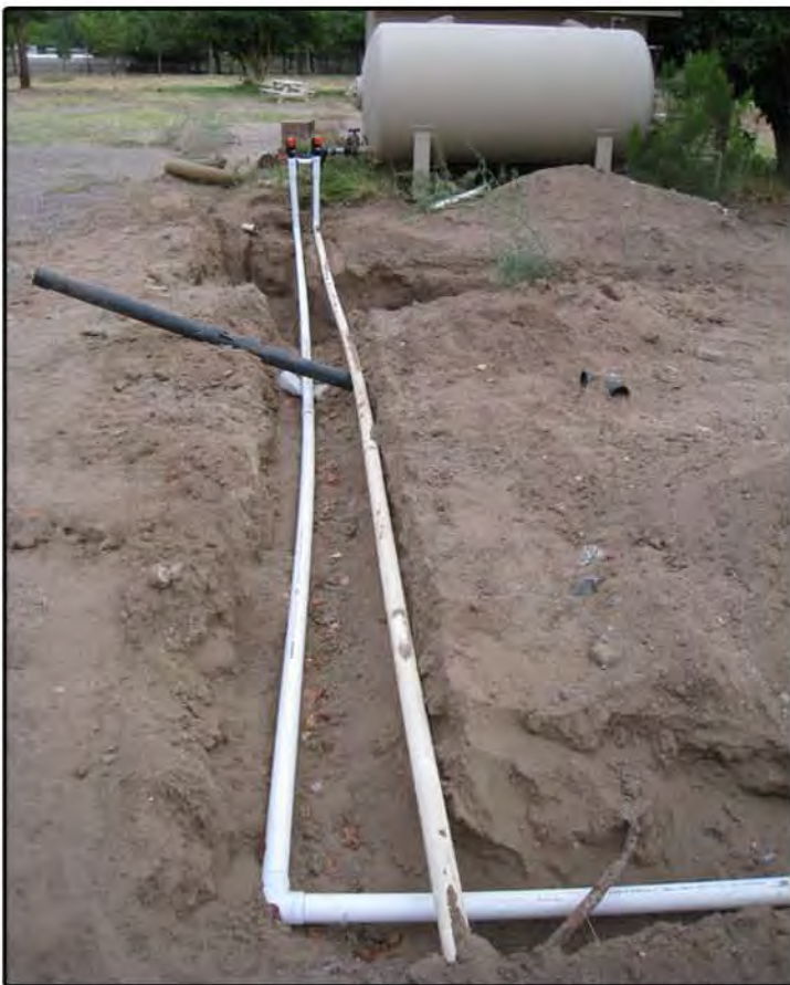
Irrigation main line connection to control valve and pressurized tank
