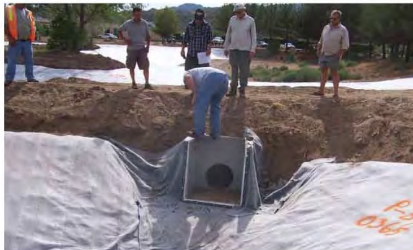
Stop log structure at the bottom of the wetland channel
