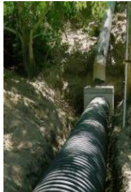
Old culvert connected to a sediment collection box and a new culvert section
