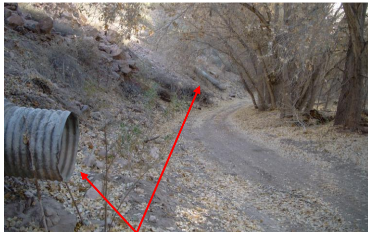
The arrows point to two of the culverts prior to the project implementation, ending at the eastern edge of the ranch fields
