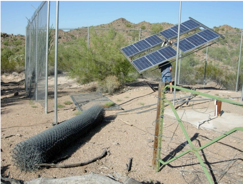
Fencing not completed to protect solar array and pump. August 2007.
