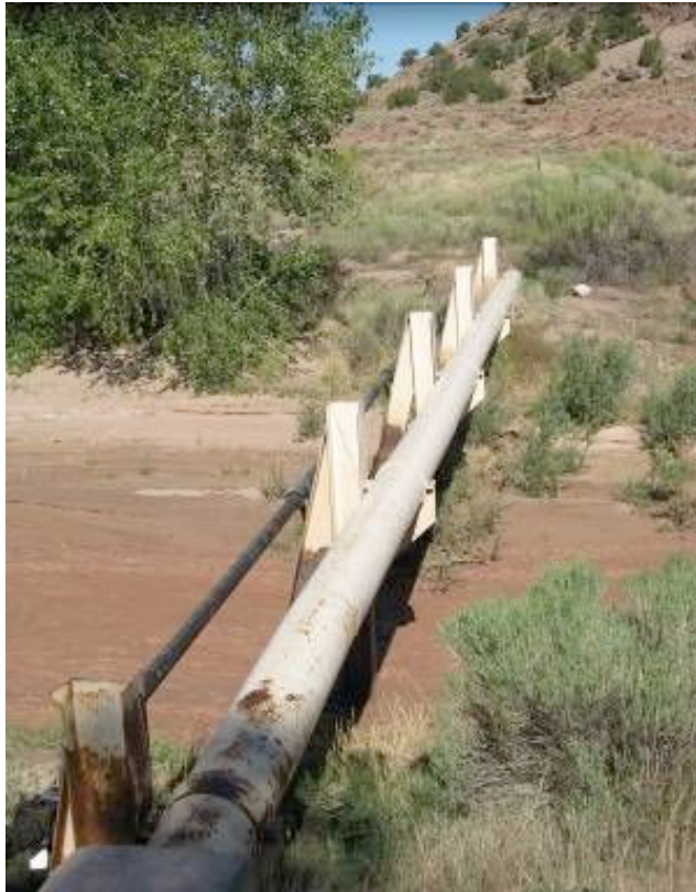
Conveyance pipe (black) crossing Pueblo Colorado Wash from sewage lagoons towards NPS. October 2007.
