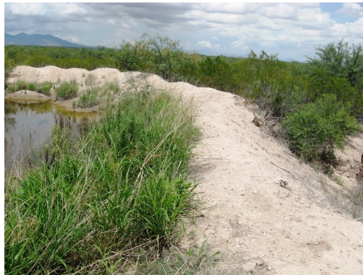
Water and sediment control basin (earthen berm) constructed to mitigate advancing headcut . July 2007.
