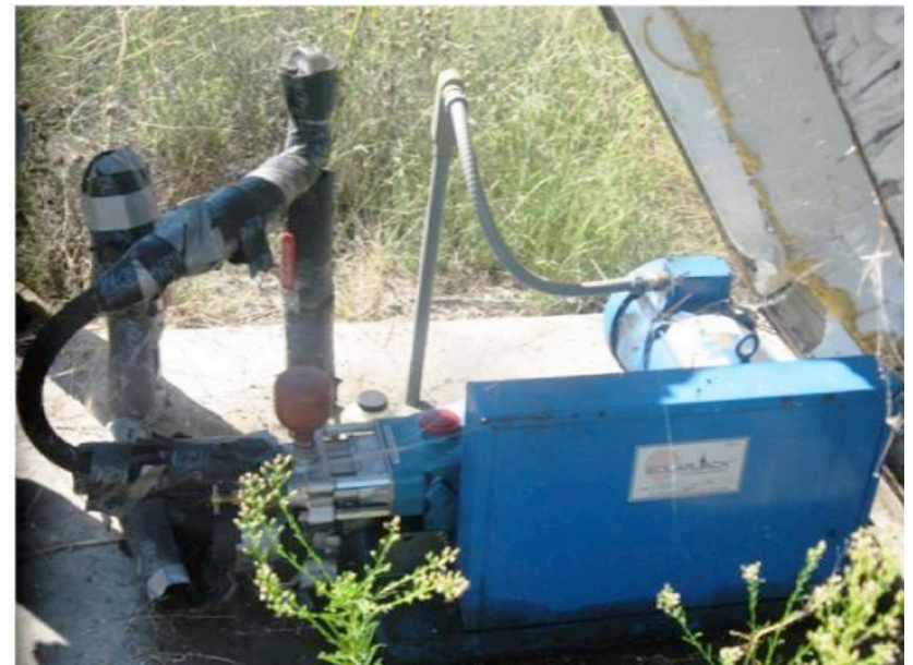
Grundfus pump September 2007.
