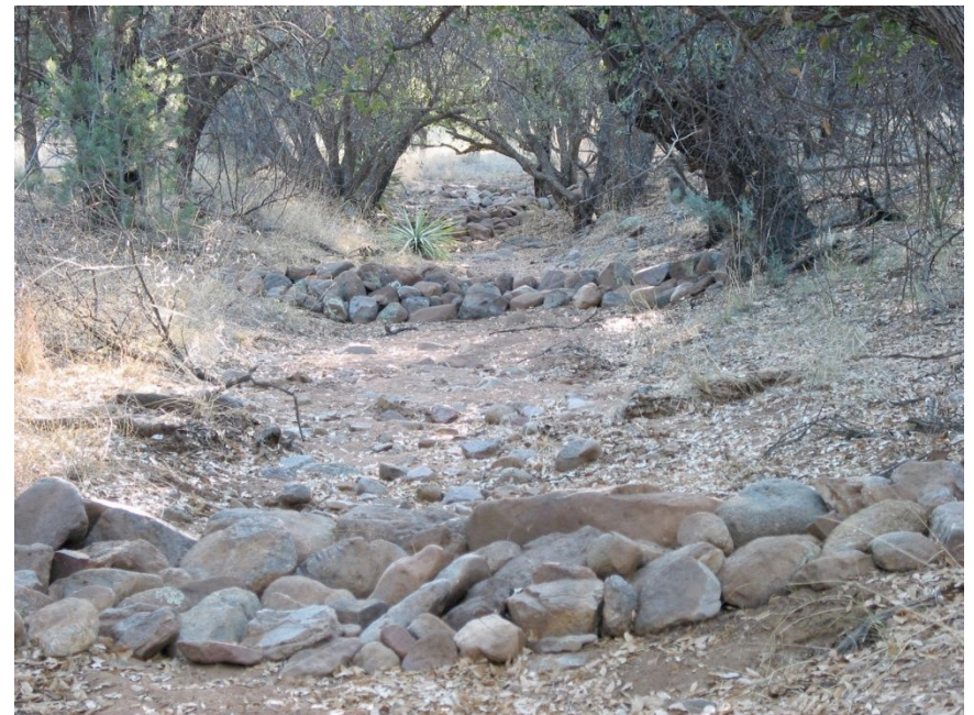
Hundreds of low rock structures were installed to capture sediment, dissipate energy, and increase infiltration. 2004.
