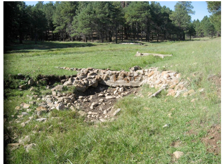
Lessons learned: drop/spillway structure below tank starting to fail.
