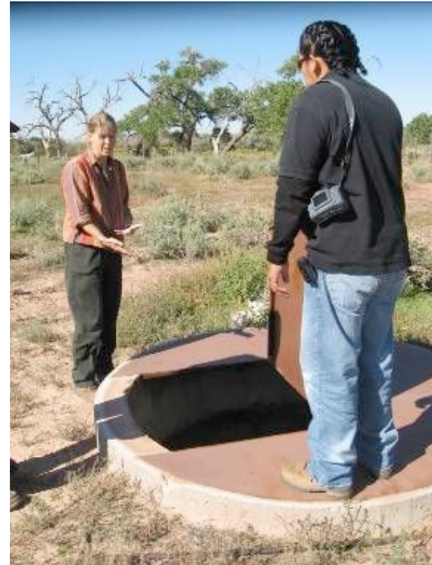
Collection reservoir at Hubbell Trading Post. From here water is delivered to gardens or riparian terrace. October 2007.
