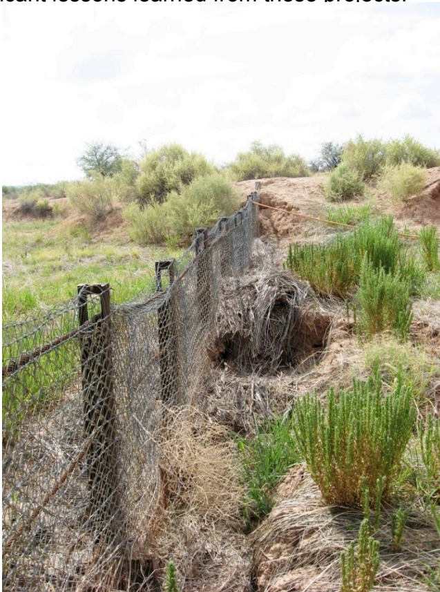
Sediment build up behind a remaining railroad rail sediment trap structure. July 2007.
