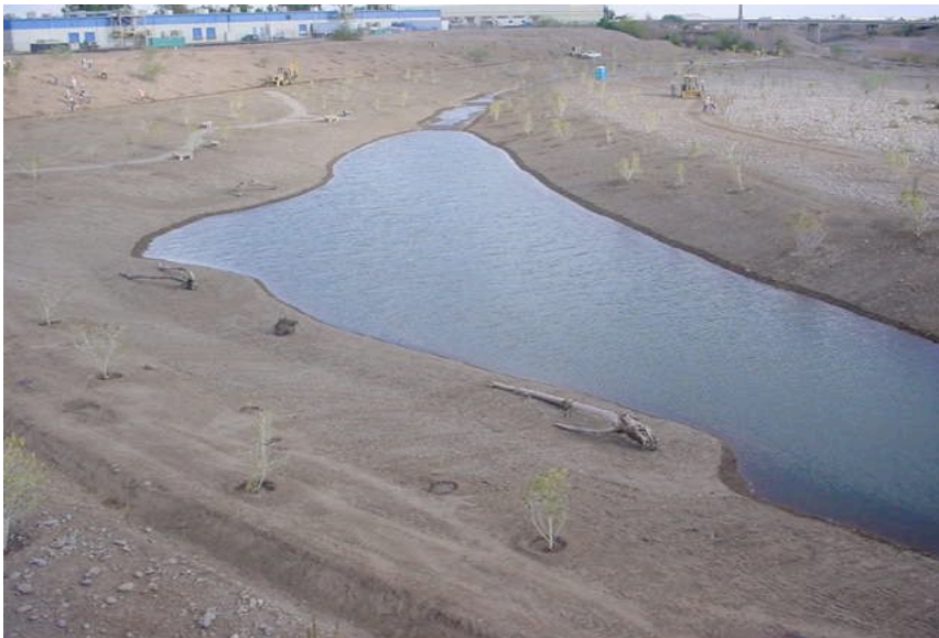
Trash was removed and project area was recontoured and backwater wetland created. Supplemental irrigation was used to establish native plantings. January 2003.
