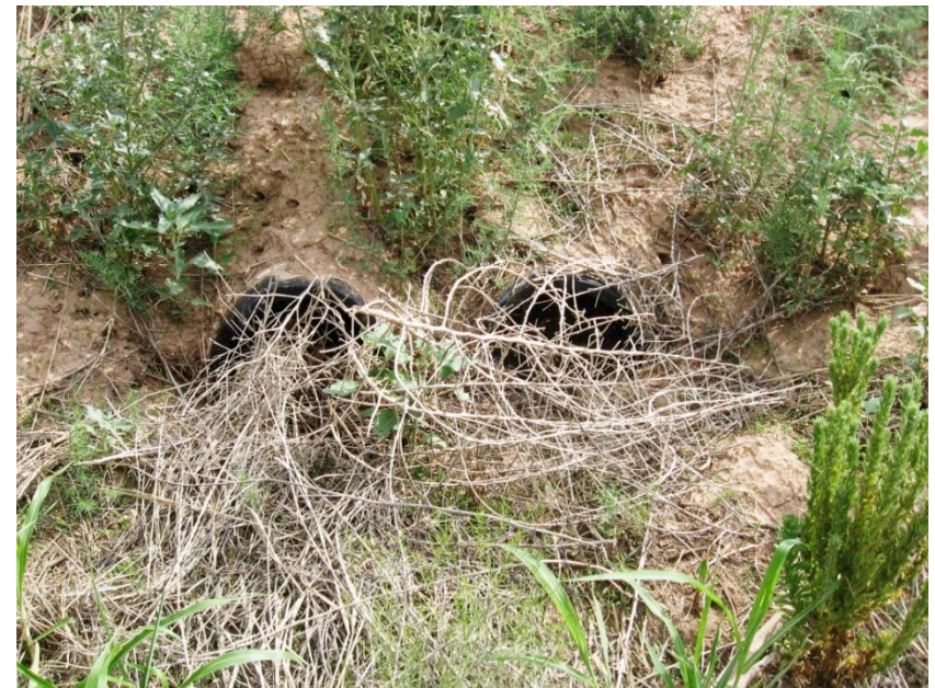
Culverts in the breached dirt berm. View from the upstream end of culverts. July 2007.
