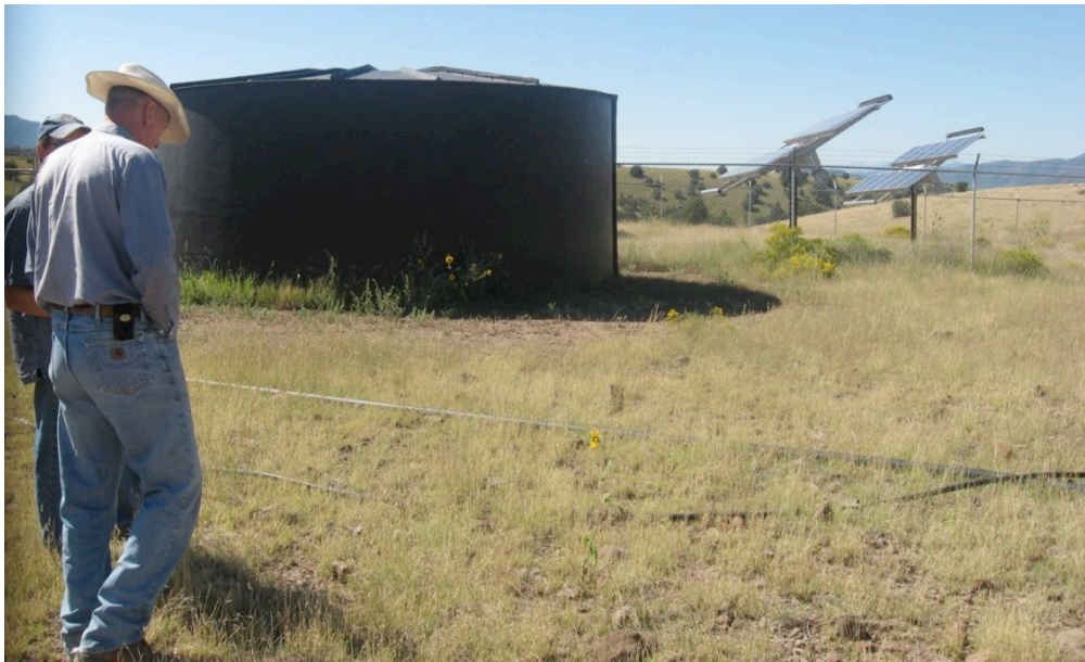
Water holding tank and solar array and pump. September 2007.
