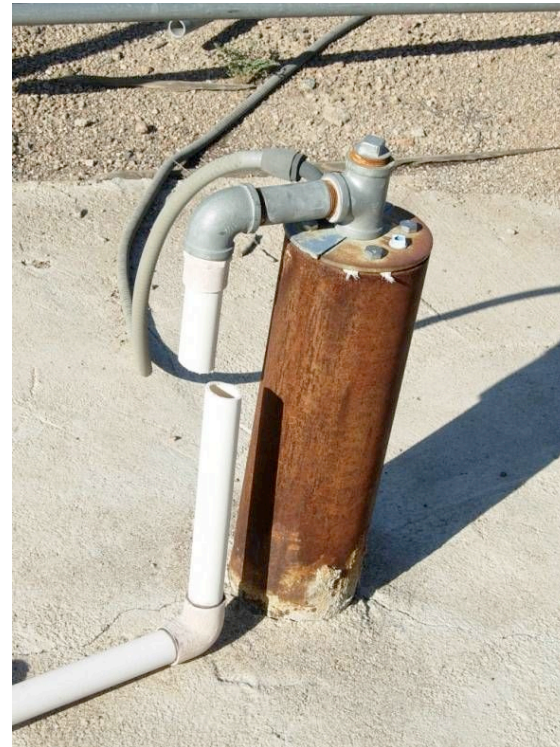
Disrepair of pump and pipeline. August 2007
