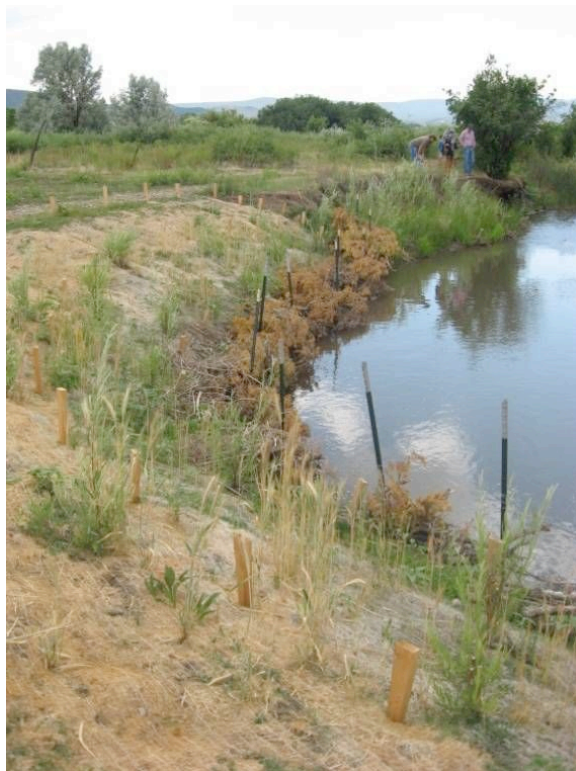
Slope bank with newly planted vegetation and Christmas tree revetments. Note erosion control fabric and stakes. 2007.
