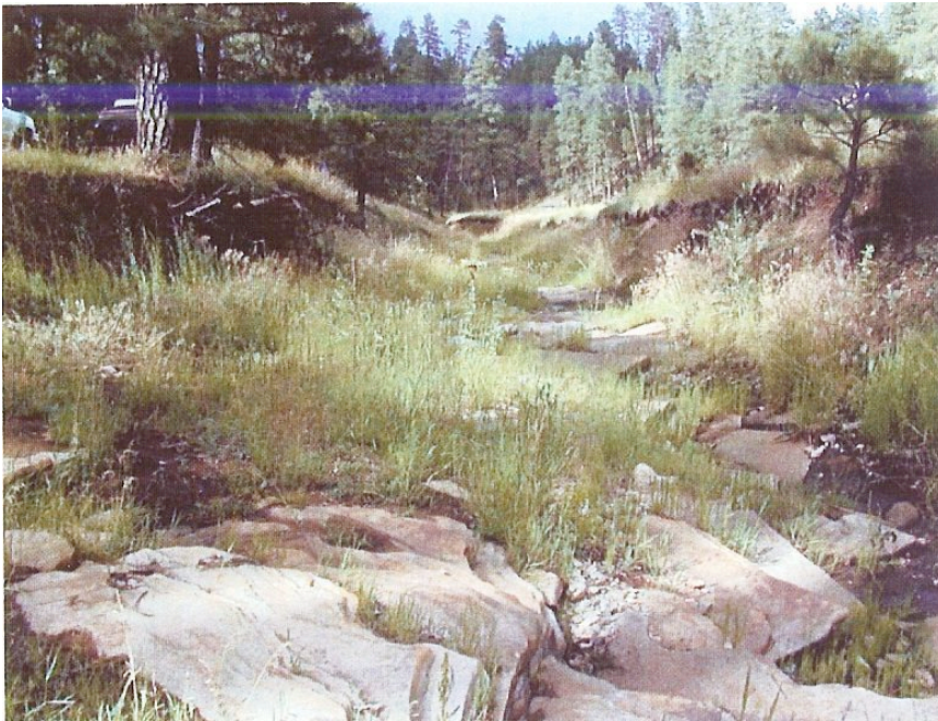
Clover Springs pre-restoration. Notice erosion and depth of gully.
