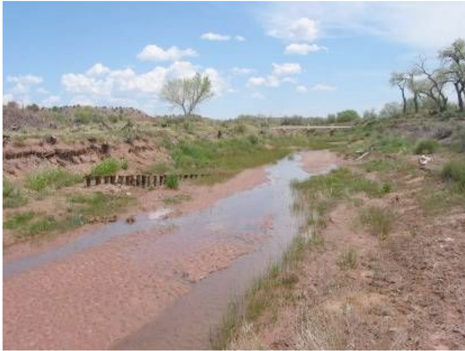
Figure 13. Post vane used for bank stabilization at the Demonstration Enhancement of Pueblo Colorado Wash at Hubbell Trading Post and Continued Enhancement projects (#97-029WPF and #00-104WPF) (left-hand side of picture).
