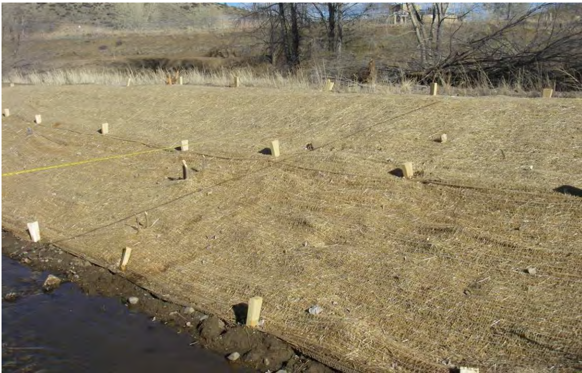
Figure B 18: BEHI 4 bank photo, April 2009
