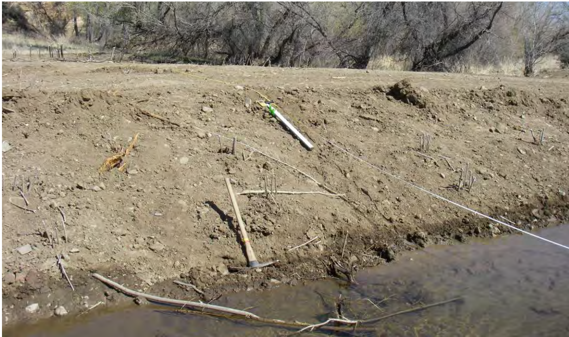
Figure B 24: BEHI 5 bank, April 2009.
