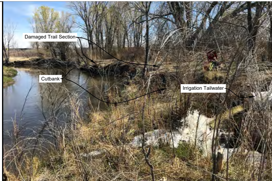
A Cutbank, Irrigation Drainage, & Trail Damage
