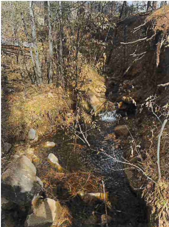
Figure 7: First unnamed tributary of Chase Creek and site of one bridge installation
