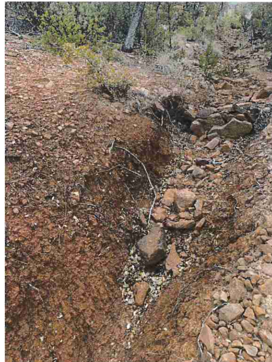
Figure 5: Riff and erosion such as this is not uncommon on sections of trail will be decommissioned and rehabilitated.
