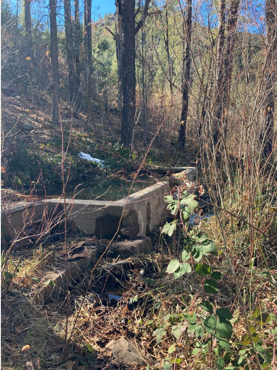
Photograph 1: Photograph of the existing spring box. The spring box leaks in multiple locations.
