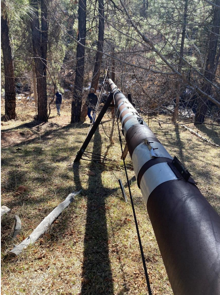
Photograph 2: Photograph of current piping that delivers water from the spring box to the pond. The pipe is elevated above Christopher Creek.
