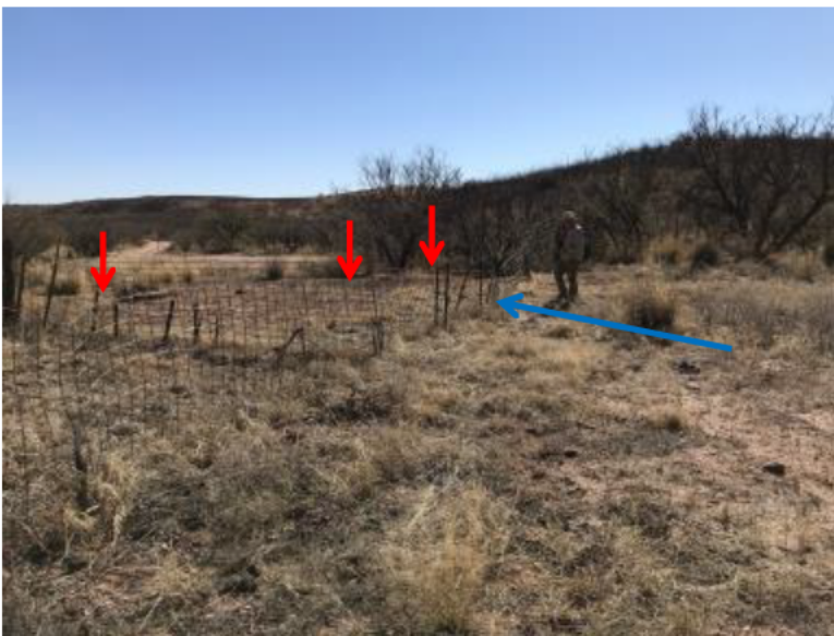
Filled in dirt tank in historic valley floor (GPS point 11): Blue arrow points in down-valley direction. Three red arrows approximate where three headcuts are eroding the historic berm. It would be advantageous to direct flows away from this filled in dirt tank so that sediment contributions might assist in maintaining the historic bajada below here.
