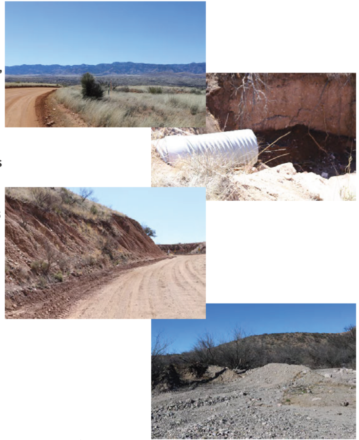
From Top: Bonita Klondyke Road; Culvert Exacerbating Downcutting; Cutslope Rill Erosion; Agradation at Klondyke Wash
